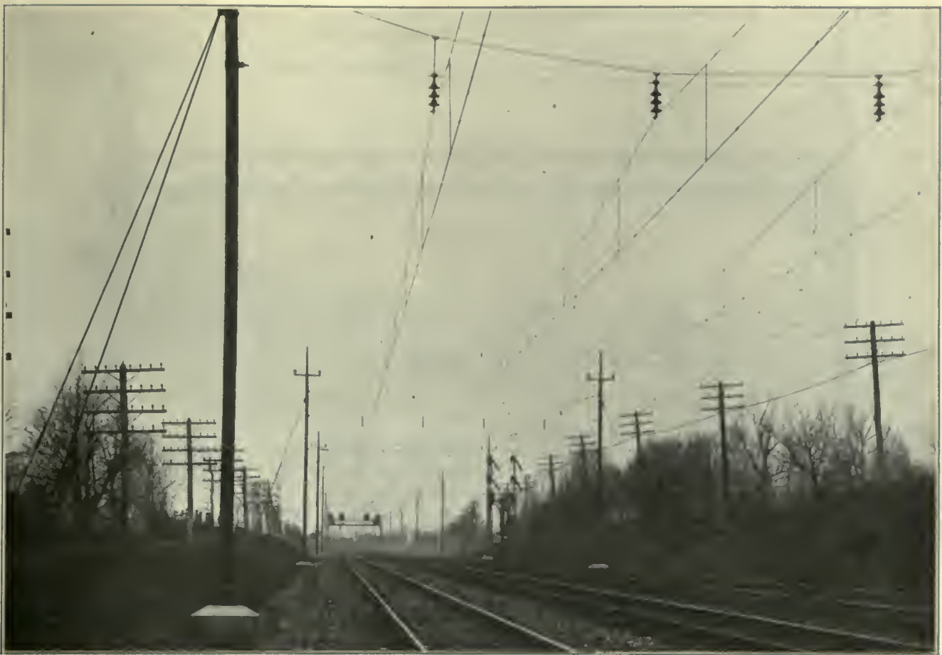
FIG. 515. OVERHEAD CONTACT SYSTEMS. Single Catenary Overhead Contact System on Tangent Track. 11,000-Volt Single-Phase Main Line Construction, Pennsylvania Railroad, near Philadelphia, Pa.
